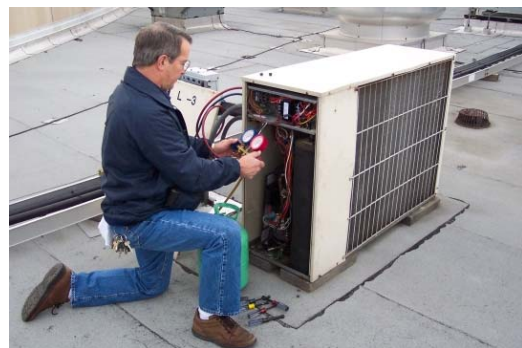
HGS Staff performing maintenance
